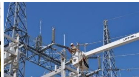
Substation Up to 765kV
