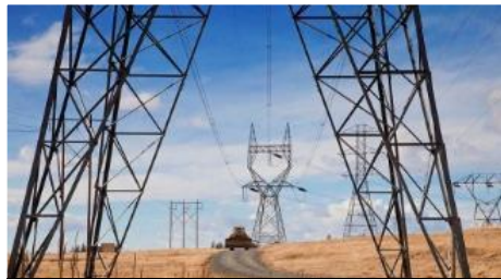
Transmission Up to 765kV
